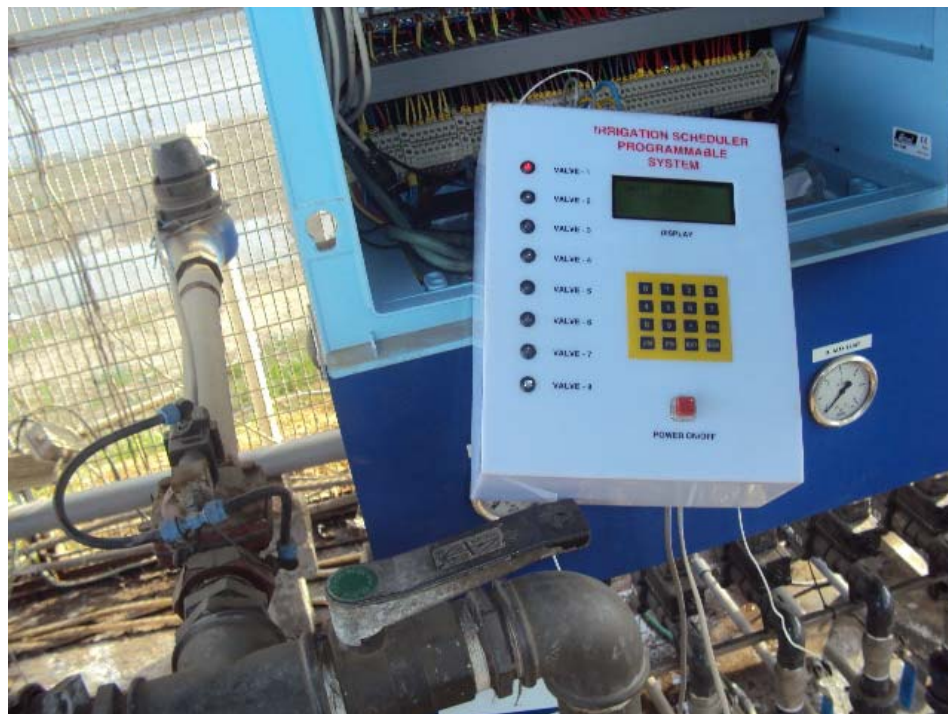
Fig.3 Scheduler connected to field solenoid valve (above) and irrigation & fertigation systems (below)
